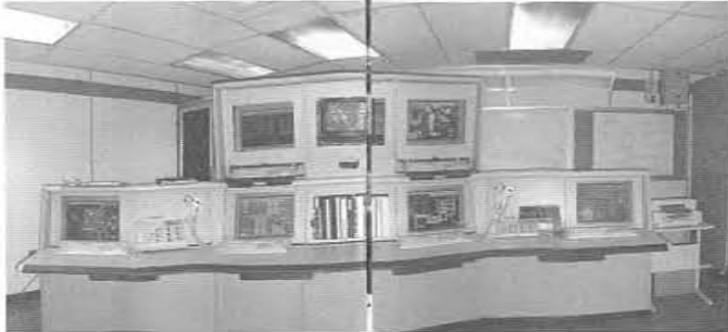
1985: The Central control room is built. The pneumatic instrument and control system is replaced with digital electronics.
