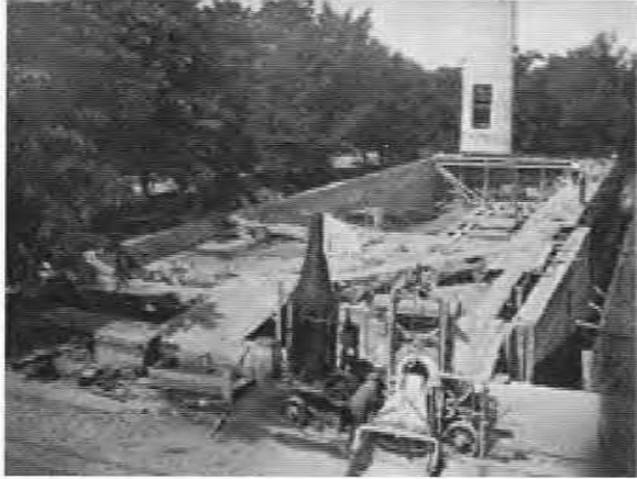
1921: The foundation is laid for the new power plant at the corner of Fifth Street and Stewart Road.
