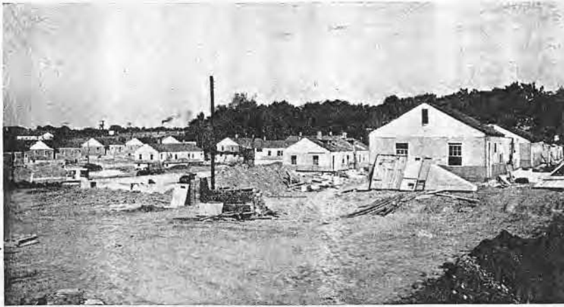
Shown here in the process of construction are a number of the faculty housing units. There will be 90 units in the Faculty Housing, located in an area southeast of Defoe Hall. Each unit in the faculty home consists of two bedrooms, living room, kitchen, a bath, and a full basement.
